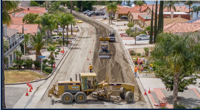
Longhorn Dr. - Progress (from Big Range Rd. South intersection to before Red Barn Pl.)
